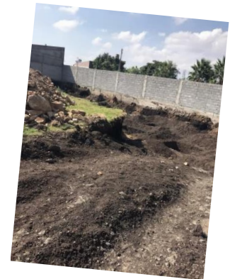
Construction photos as ground preparation began for the new 11 th & 12 th grade structure.
